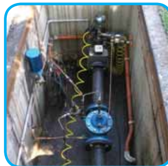
Smart technology reduces leaks and bursts and ensures the water pressure meets the demand.
