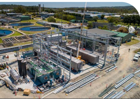
The wastewater treatment plant will benefit from $224.7 million in essential road and water infrastructure spending.
