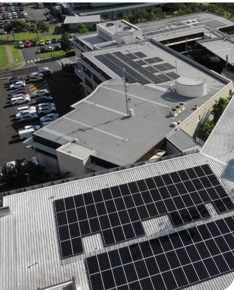
Solar panels on top of Logan City Council Administration Centre building.
