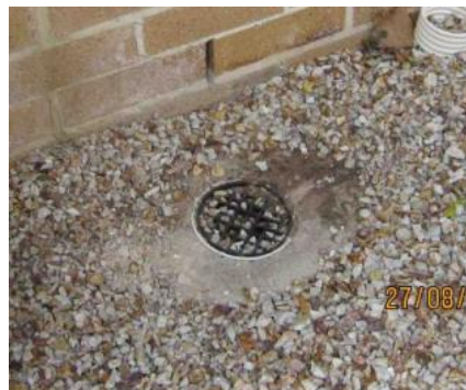
ORG not raised above surrounding ground allowing surface rainwater into the wastewater network
