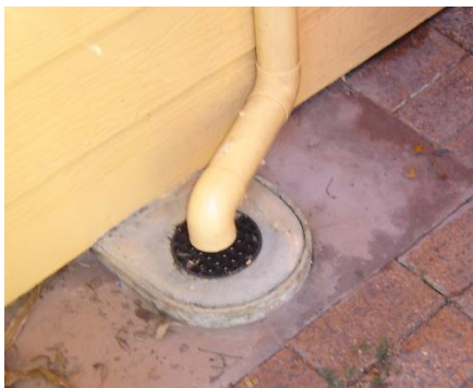
A roofwater downpipe draining to an ORG allowing rainwater into the wastewater network
